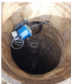
Sewage pit level monitoring
